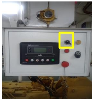
Gambar 7. Panel Generator AC
